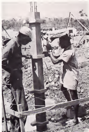
Peace Corps volunteer Private Willie M. Wilkerson (left), instructs a student in the use of concrete molds in West Cameroon. Wilkerson, who served two years as a Peace Corps engineer and instructor in the African nation, is currently undergoing training with Company D, First Battalion, First Engineer Training Brigade at Fort Leonard Wood. (U.S. Army Photo)
