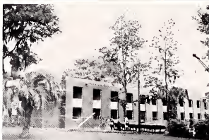
The Women's Dormitory is one of several buildings now under construction. The dormitory will accommodate 160 women students.
